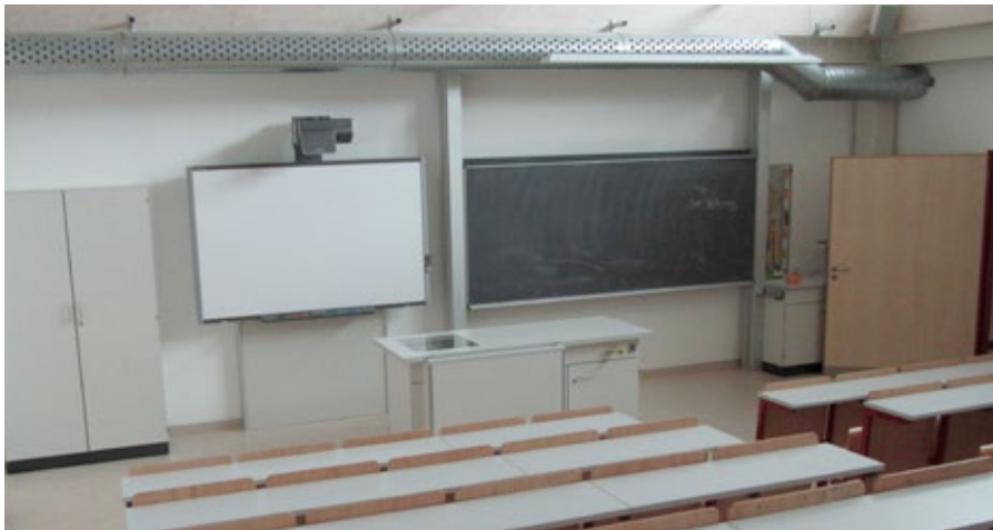
Theben Amun 716 R CO 2 sensors control and control the ventilation in classrooms to exactly meet the requirement for fresh air.
